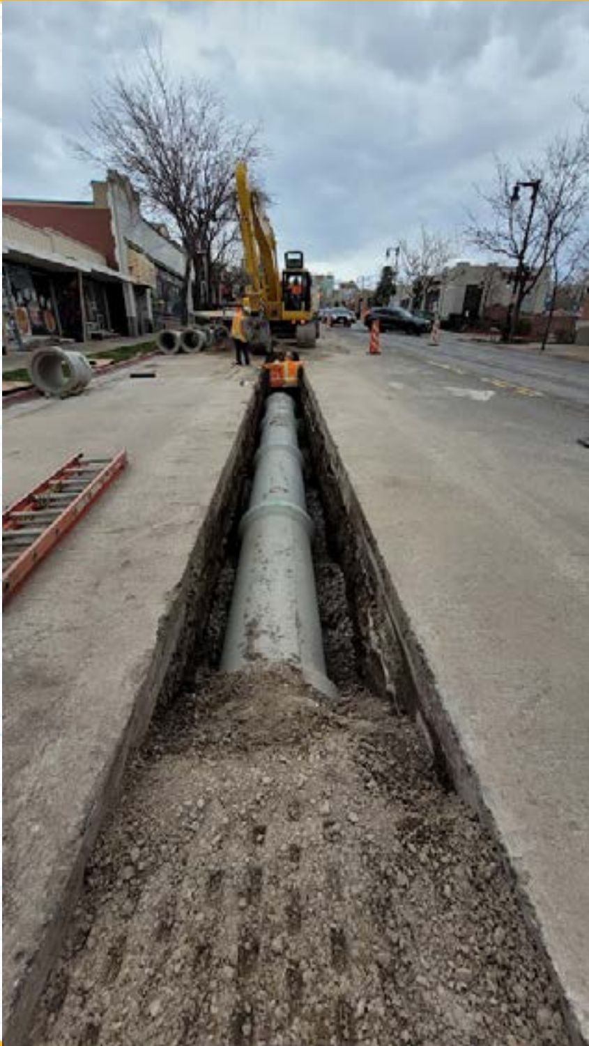
The 2100 South Sewer Upgrades project, completed in September 2024, is one example of targeted asset replacement.
