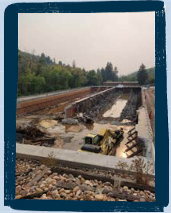
Demolition of the flocculation and sedimentation basins at City Creek Water Treatment Plant September 2024
