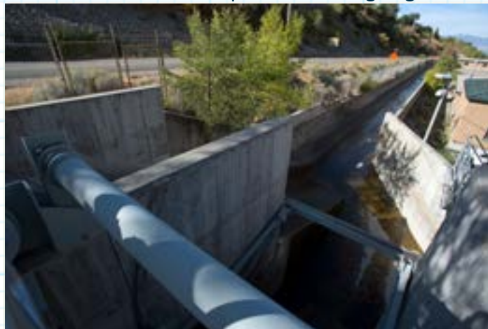
Small projects, such as replacing the concrete creek channel pictured above, will extend the lifespan of the BCWTP until it can be rebuilt.
