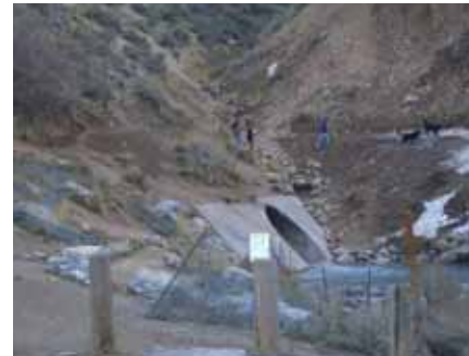
Photo 39: Dangerous user-created trail eroding into Parley’s Creek.
