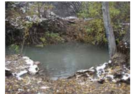
Photo 21: Turbidity and erosion.
