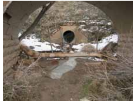
Photo 12: Two culverts for routing off-site runoff through the park. The top of the second, buried corrugated metal pipe is visible inside the archway.
