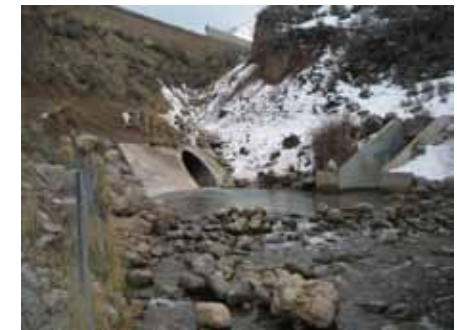
Photo 15: Outlet of Parley's Creek culvert (left side), highway drainage culvert (above it) and outlet of Terminal Reservoir (right side).
