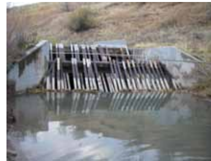
Photo 5: Debris structure at west culvert inlet.
