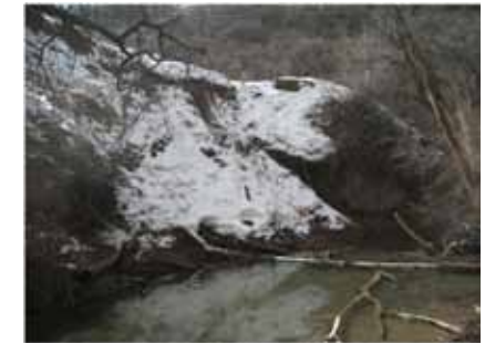
Photo 6: Erosion and debris in channel.
