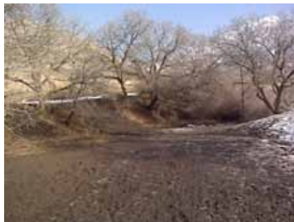
Photo 44: Poor trail design and drainage creates muddy patches and causes users to step off-trail, exacerbating the problem.
