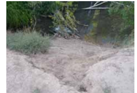
Photo 34: Dangerous eroding creek bank.
