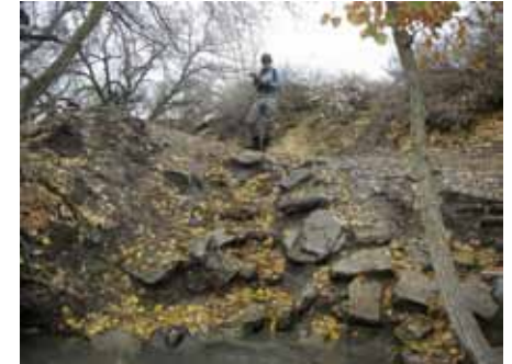
Photo 17: Bank hardening from trail and rip-rap.
