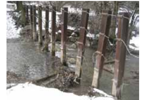
Photo 4: Debris structure west of main bridge.
