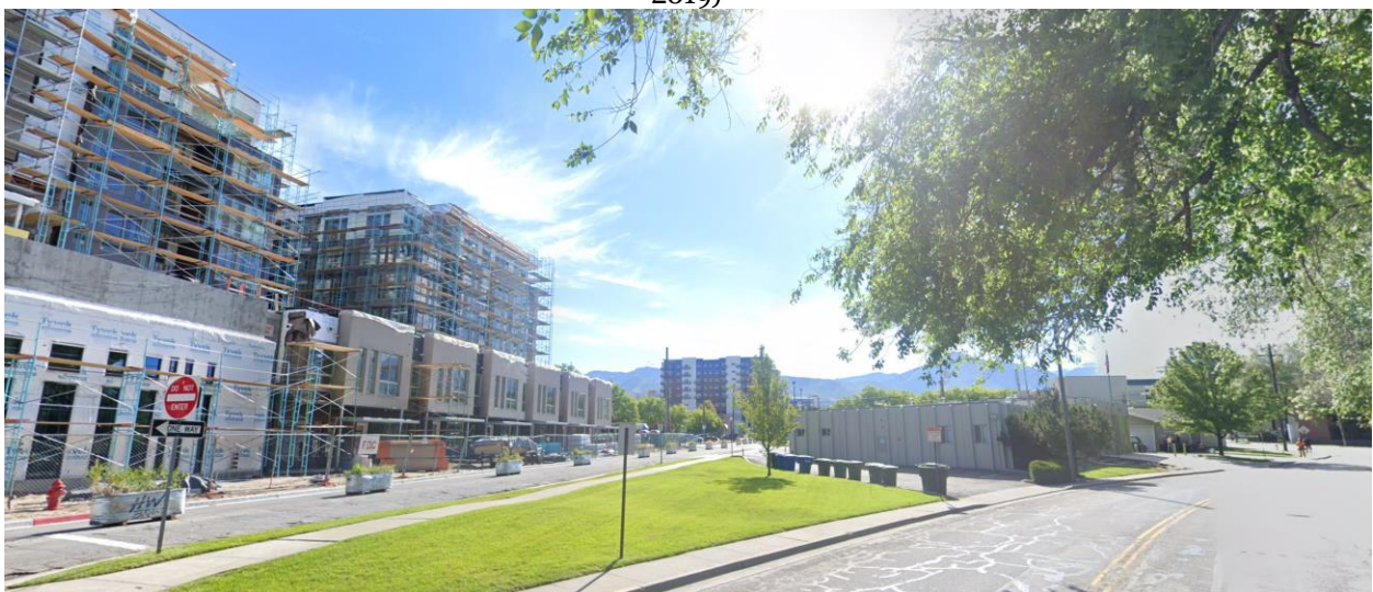
View of the west corner of the site from Simpson Ave, looking east (Credit: Google Street View, 2019)
