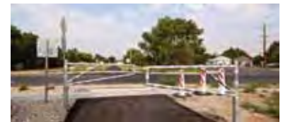
A 10-foot wide asphalt paved trail is currently in place from Redwood Road to 700 West serving both pedestrians and cyclists. Safety gates and pavement markings are provided at all road intersections. These safety gates are of concern to trail users as it creates an ease of use issue.
